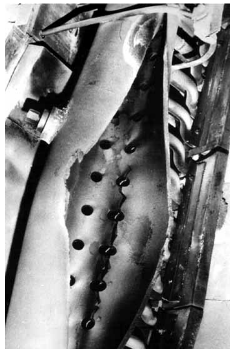
Fig. (1). A boiler header whose failure was attributed to creep rupture after failure analysis.
